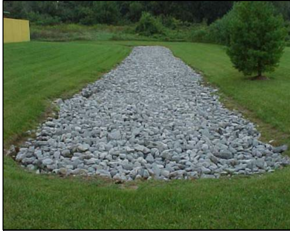
Infiltration Trench. Source: AWWA. (2019, February 1). Infiltration trench: Do-it-yourself conservation practices. Acton Wakefield Watersheds Alliance. Retrieved October 7, 2021, from https://awwatersheds.org/infiltration-trench-do-it-yourself-conservation-practices/ .
