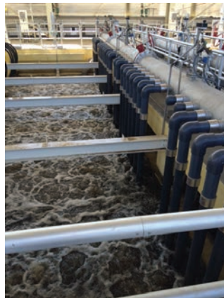
Tertiary Treatment Plant
