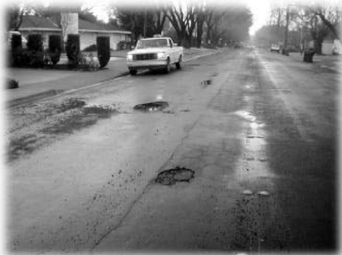
Significant potholes were evident along Sycamore Avenue this past winter.
