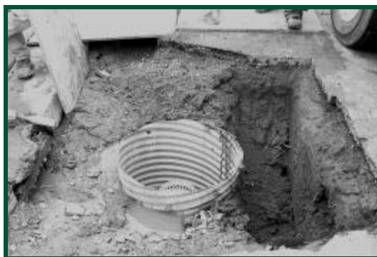
A Rockwell is installed in Modesto
